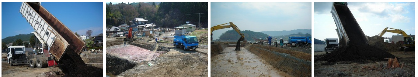
View of discharging compost and spraying EM • 1 ® into the hole of organic waste
